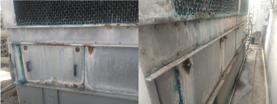
Old Panels and New Access Panels after having been coated inside and out
