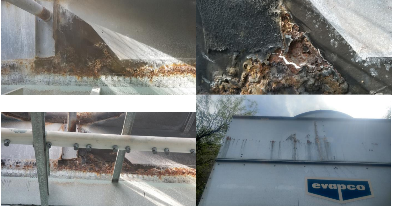
Pictures of the corroded upper deck and previous coating around compromised support before repairs.
